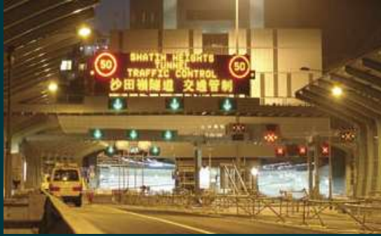
Traffic Control and Surveillance System
