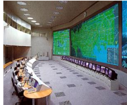
Traffic Control Center
